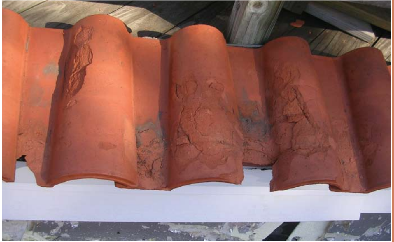
This tile on a New York school was imported from Italy and failed after 8 years.
